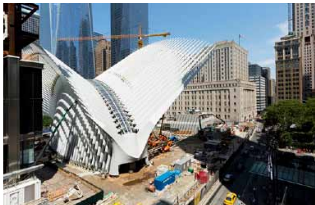
The World Trade Center Transportation Hub, designed by Spanish architect Santiago Calatrava, is under construction in New York.
