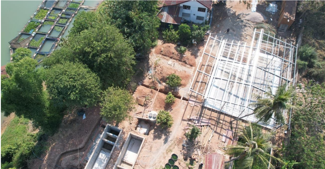
Construction of the fish processing plant at the site of Verkhnam Cooperatives
